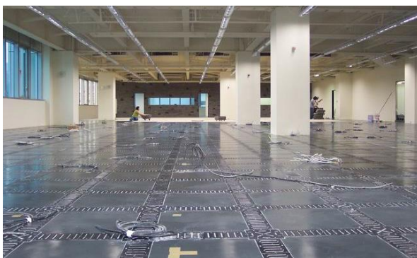
Cables routing inside the Cable Trenches and extending through any point of the floors
