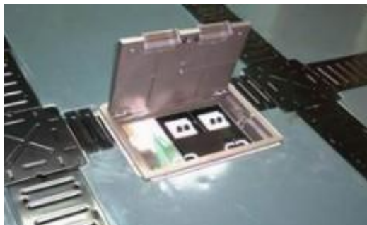
To accommodate large size floor box - Cut at side of the panel (count in the Cable Trench width) and installed at the trench,.
